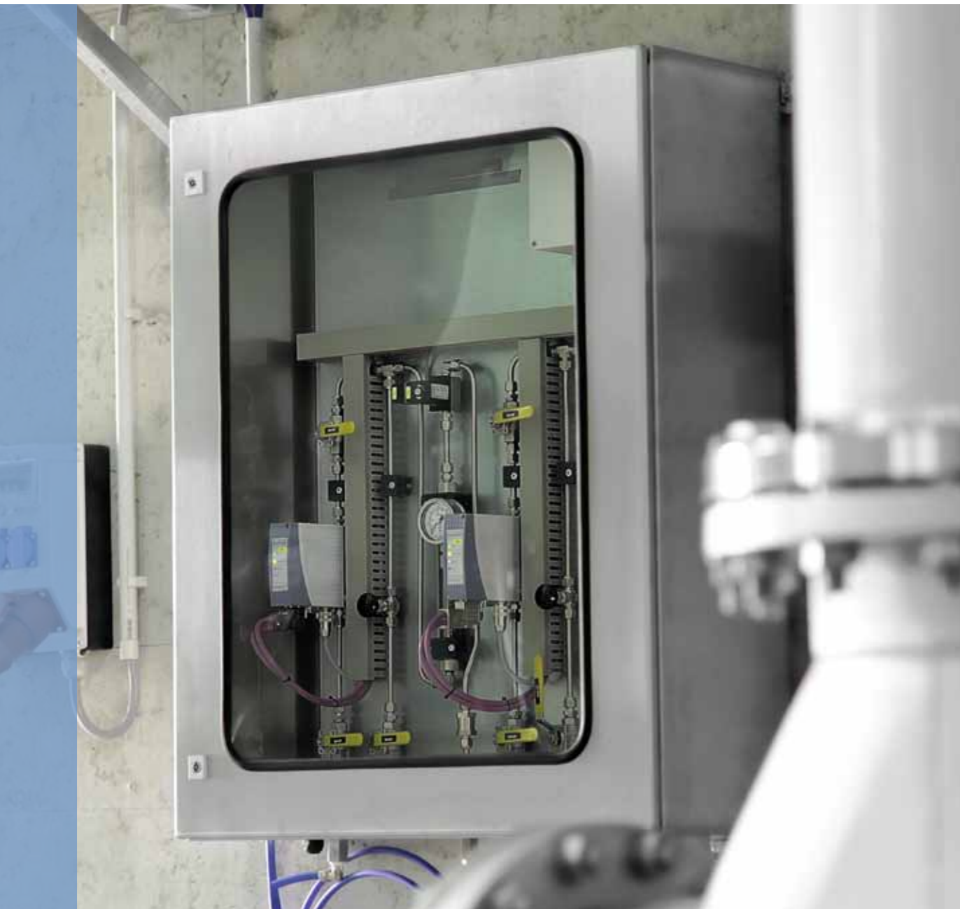
Oxidator box from Bürkert: Two-channel system in Everswinkel Municipal Utilities Waterworks
