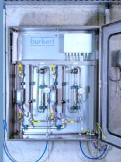
Bürkert oxidator box – inside view of the Everswinkel Municipal Utilities Waterworks
