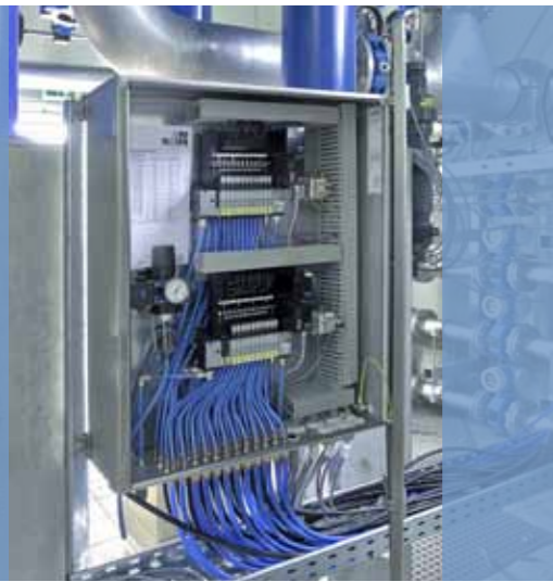
Bürkert pneumatic cabinet for filter control
